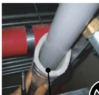
Loose fitting wrong insulation
